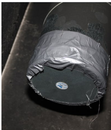
Figure 10: Completely sealed closet exhaust duct
