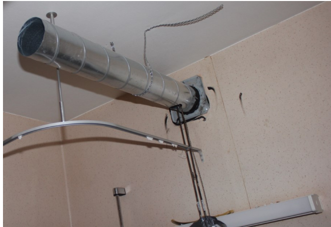
Figure 14: Exhaust velocity and temperature measurement - Bathroom
