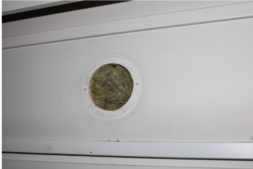
Figure 8: Supply vent in the living room
